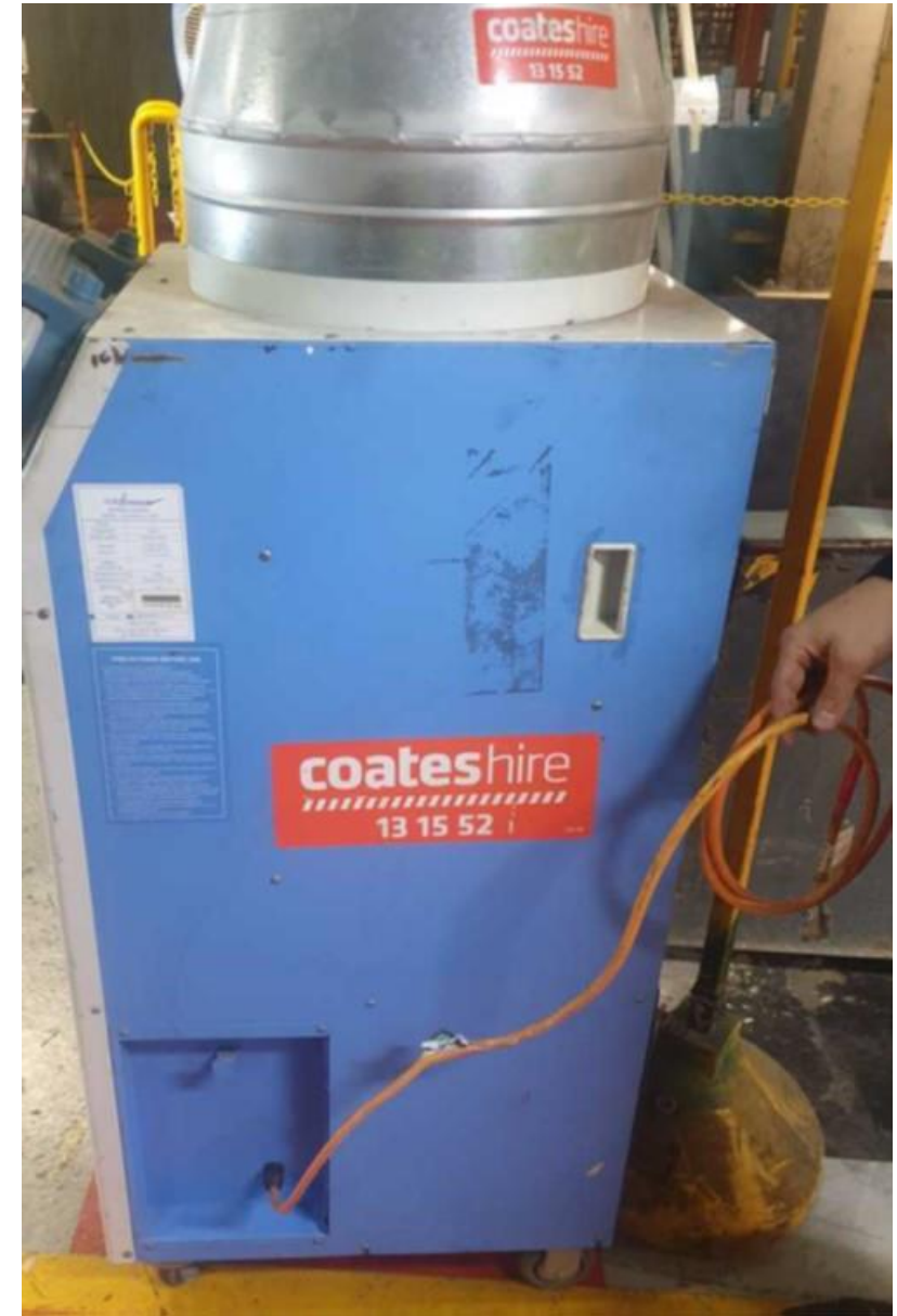
The portable air cooler with the damaged lead
