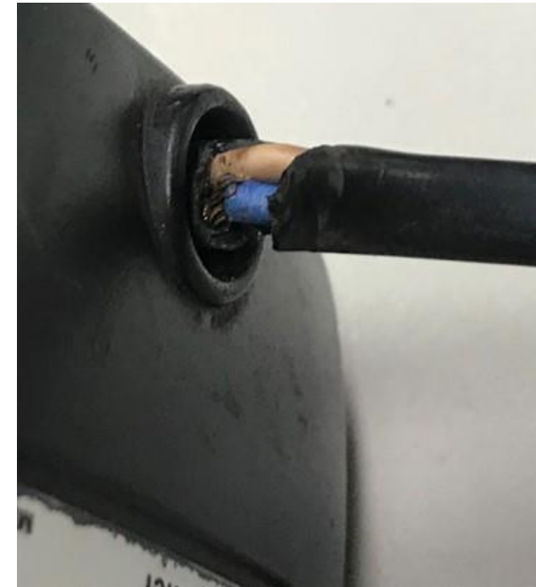
Close up view of the damaged lead and exposed neutral conductor
