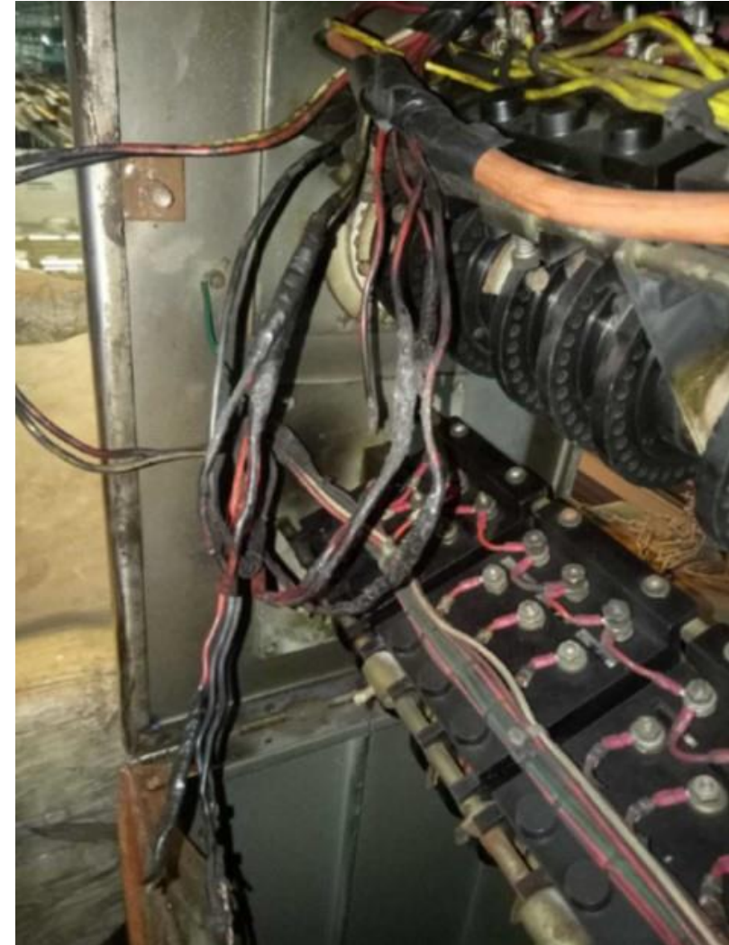
The loom opened up revealing the damaged wiring, damaged links in the cores and broken wires
