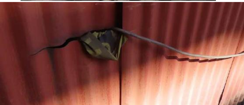
Back and front views of the cut in the wall sheeting with the lead running through it.
