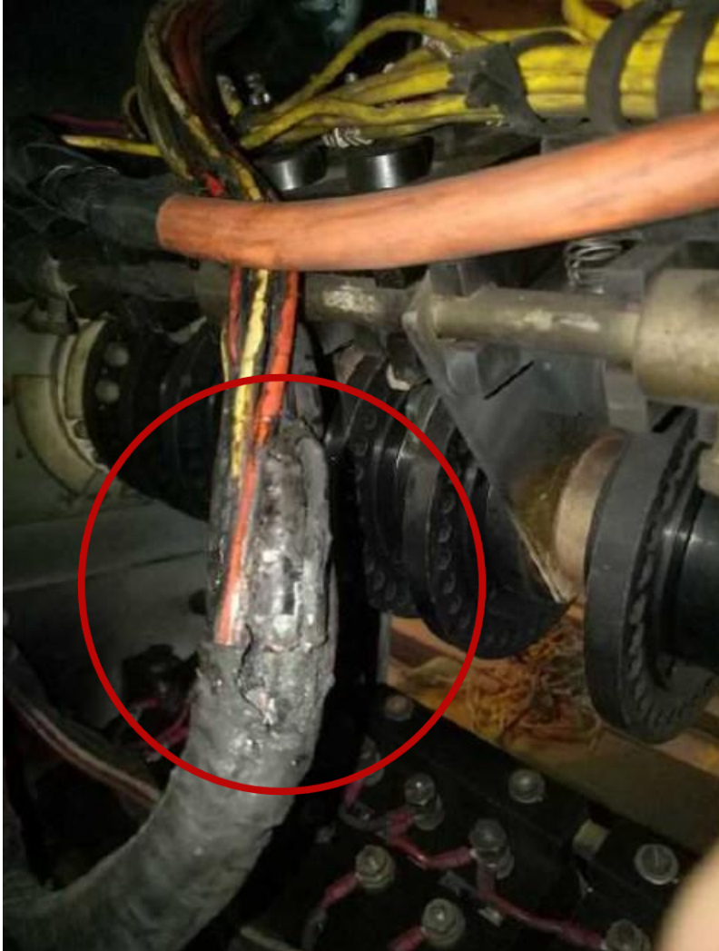
The loom of wiring inside the control desk tapped together and showing signs of heat damage
