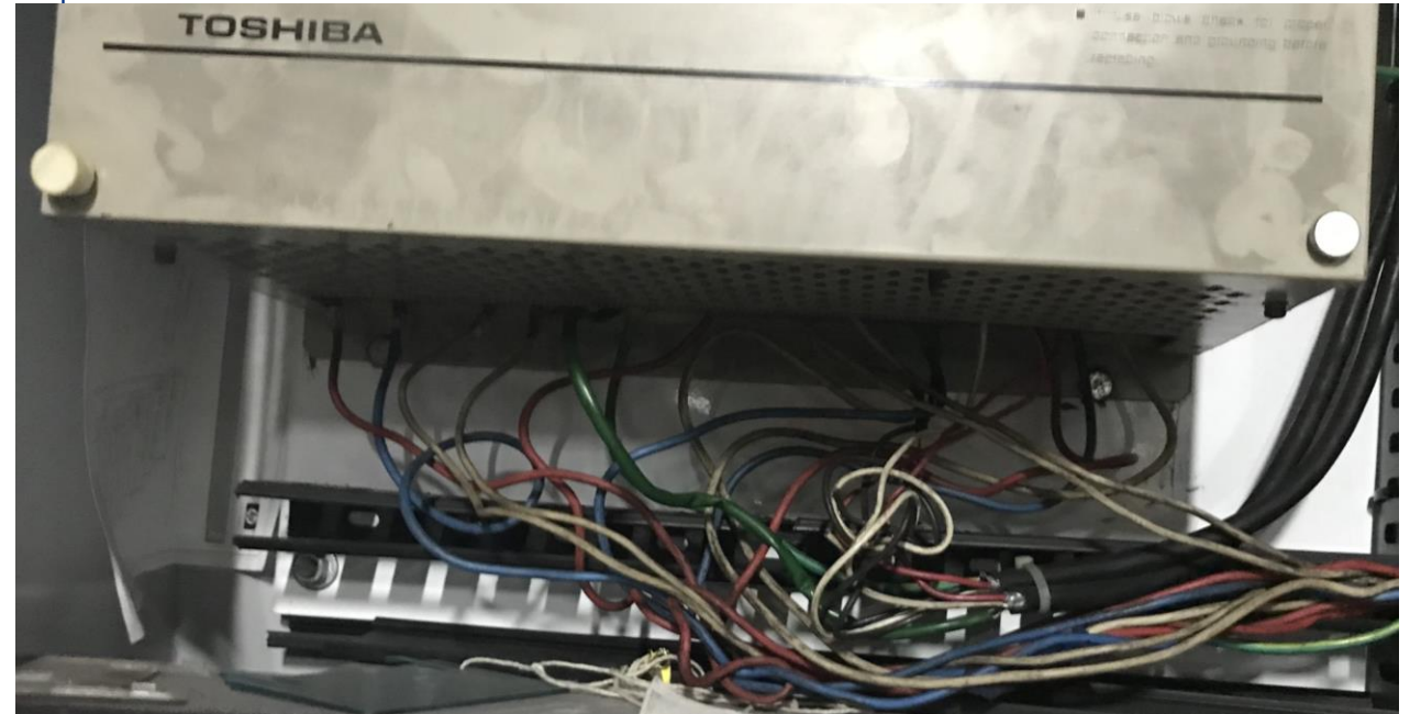
A close up of the wiring at the bottom of the drive where the electrician's left hand came in contact with the motor conductor
