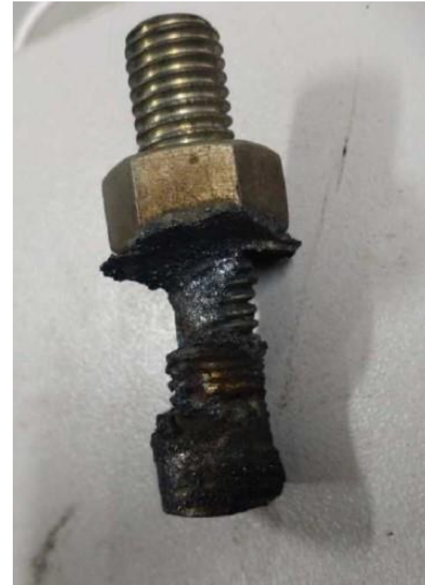
The heat effected bolt with the heat end melted round to allow bolt to come away from the busbar
