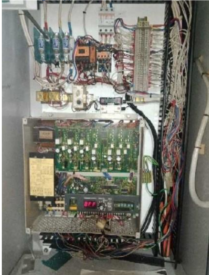
The inside of the motor starter with the drive cover removed before the VVVF was removed
