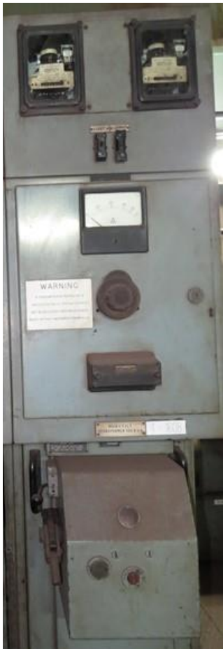
The front of the OCB breaker
