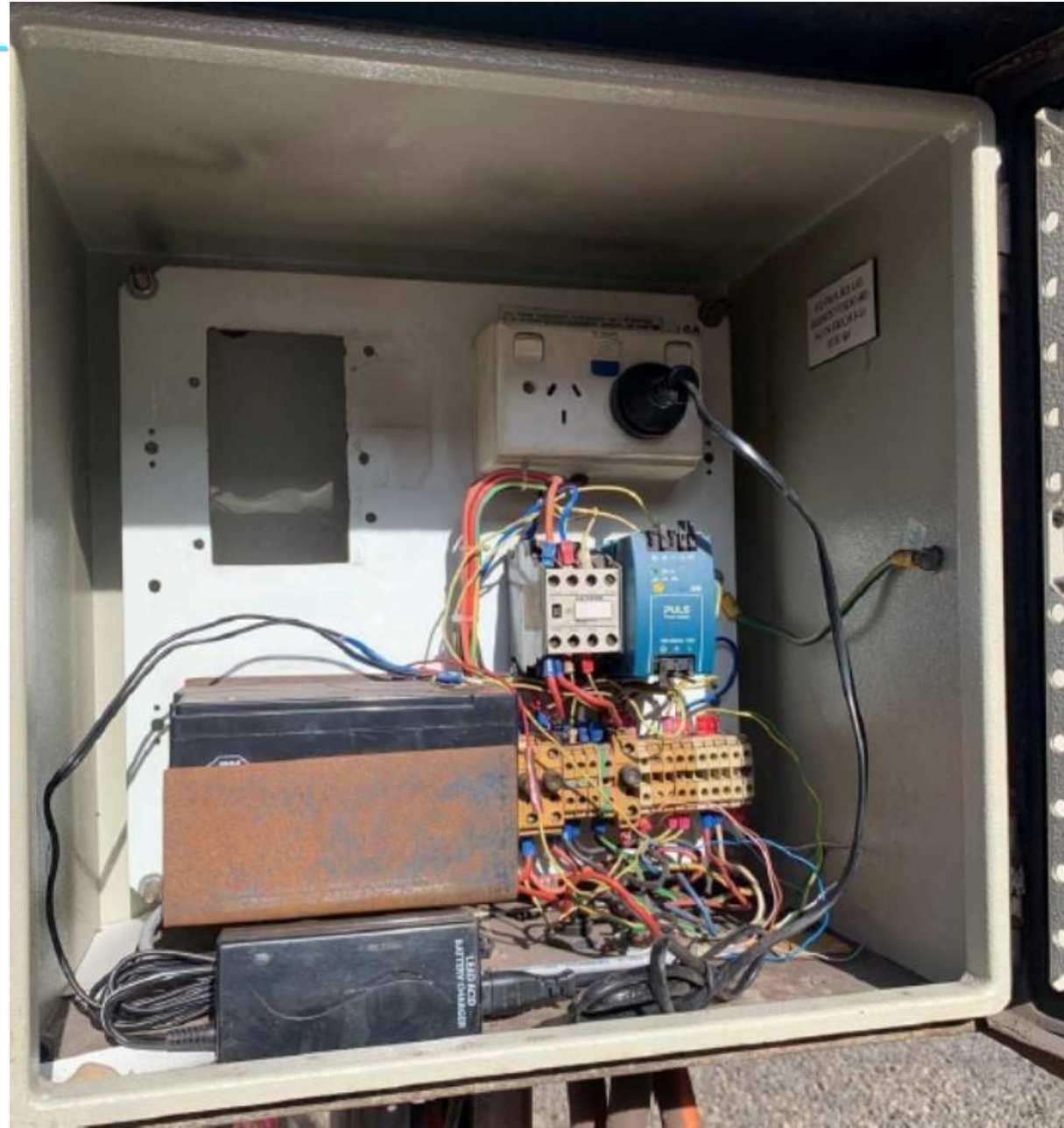
Inside the CO gas monitor j-box which was accessed by unauthorised people
