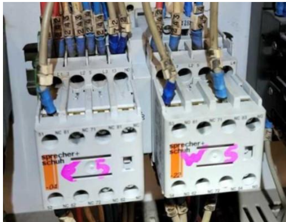
The cross travel contactors
