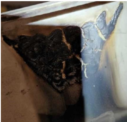
The burnt cable duct lid
