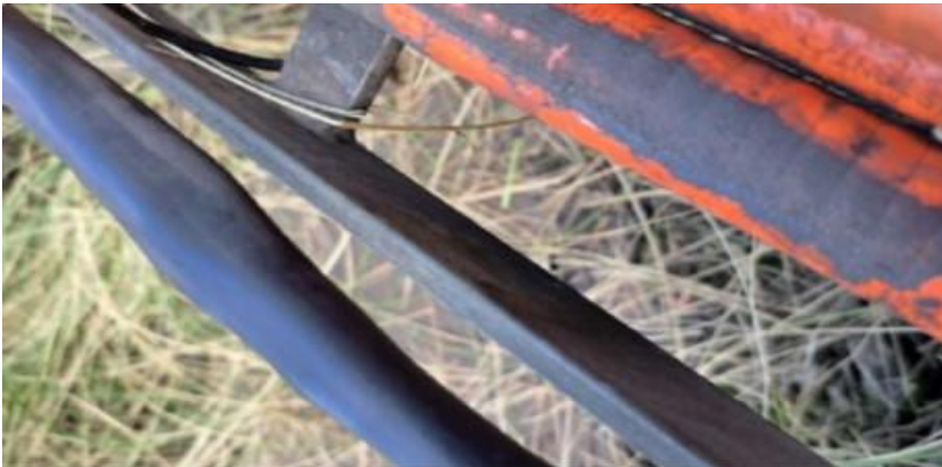
Evidence of arc marks on the side of the cable rack
