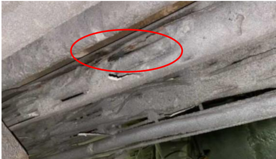
The cable racking where the damaged cables were found. Note 1, the burn marks on the rack noticed
