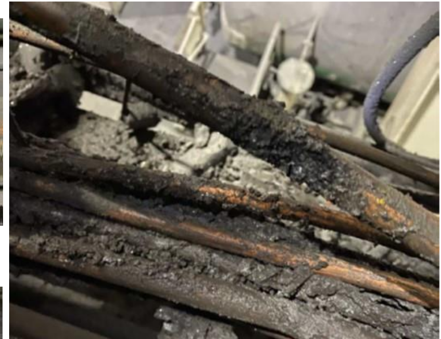
The other damaged control cable with outer sheath and inner insulation melted exposing conductors. Covered in Kish mud.
