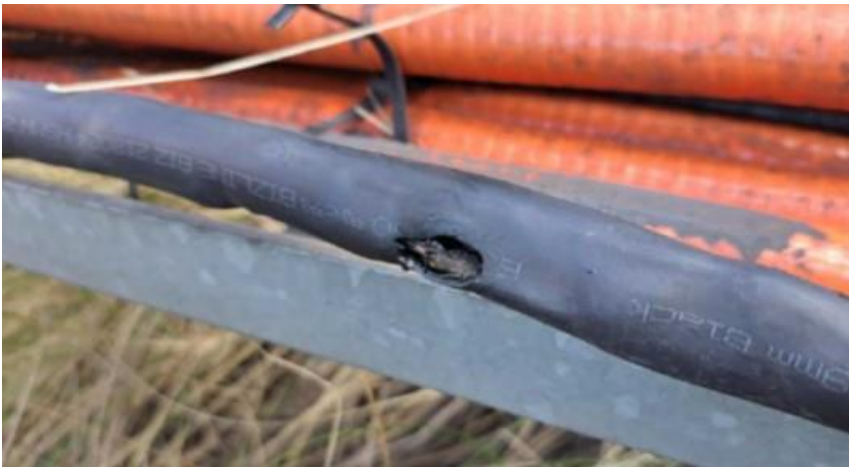
The blowout in the heat shrink cable joint
