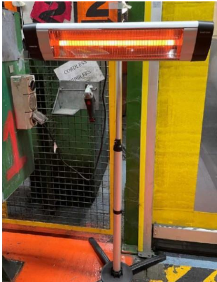
The portable heater plugged into an RCD protected outlet
