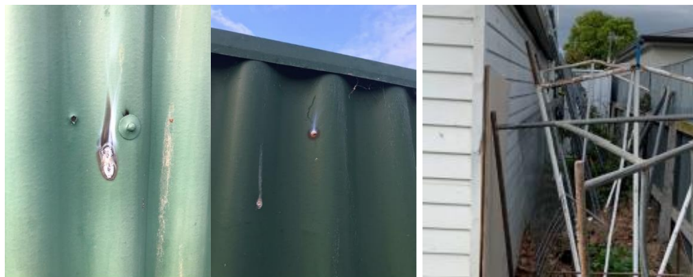
Images showing arcing on the iron fence and poles that were making contact between the fence and the storage shed.
