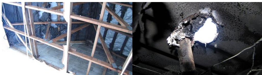
Images showing fire damage in the roof space and the hot water vent pipe that was livened.
