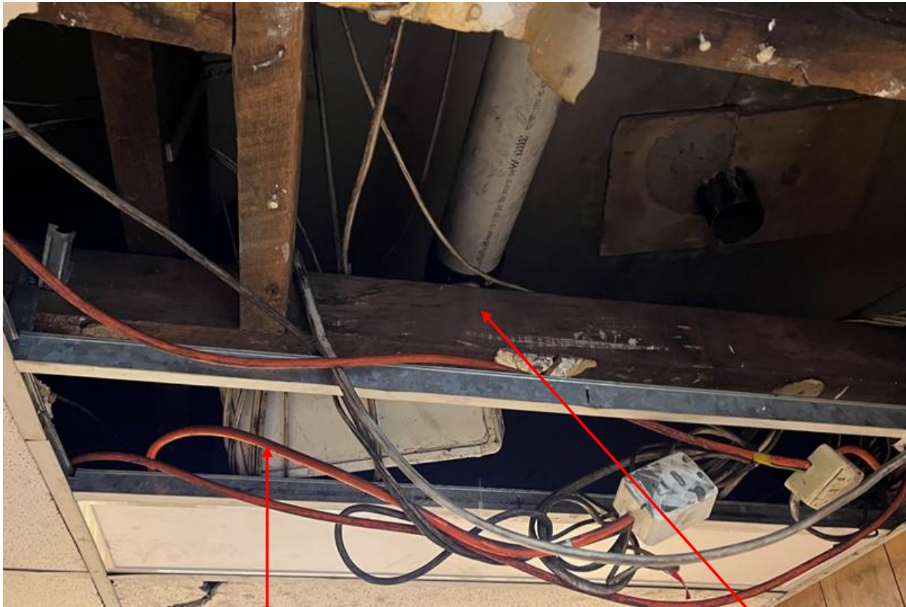
The emergency light fitting with supply cable wrapped around it
