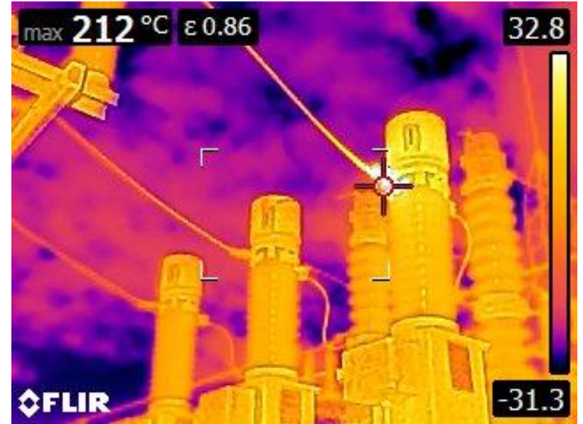
The thermal image scan clearly showing the hot joint
