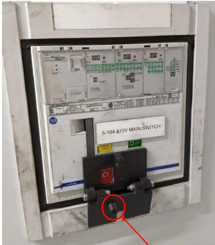
The locking mechanism at the front of the ACB. The lower flap closes onto the top section with the raised section depressing the open pushbutton
