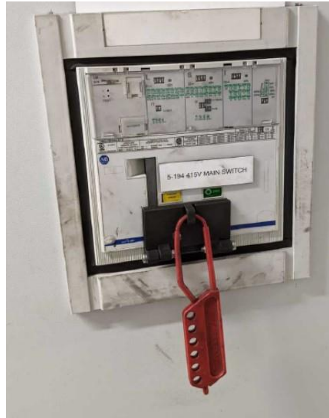
The ACB in the locked out position secured with a red plastic multi-lock device. The multi-lock does not engage the locking mechanism sufficiently to inhibit breaker close operation.
