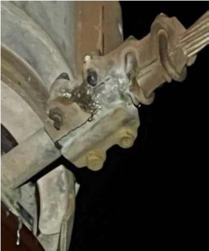
A close up of the aluminium CT connection with melting damage due to the hot joint evident
