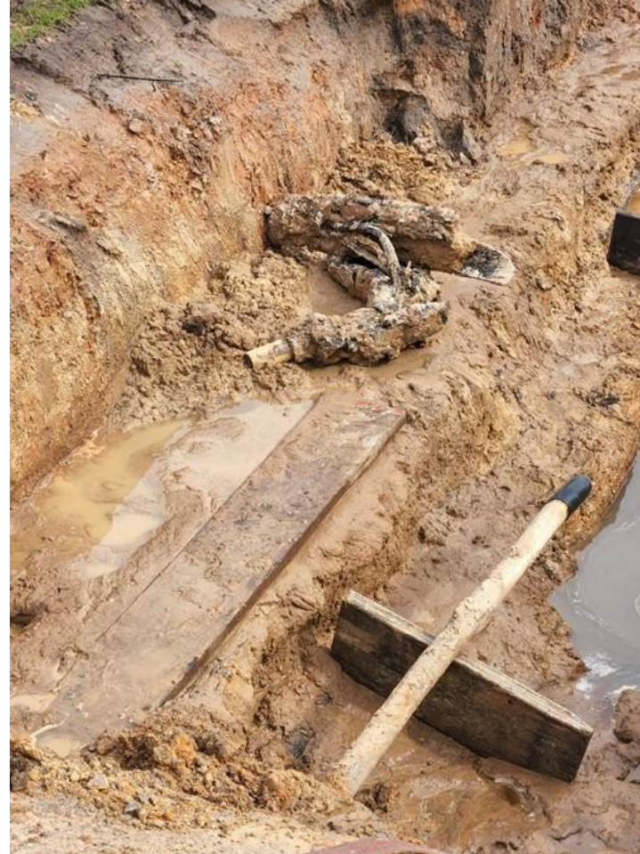
The remnants of the cable joint after it was dug up.
