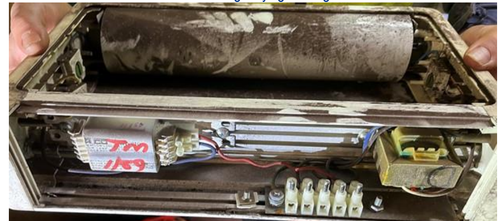
The redundant emergency light fitting as found
