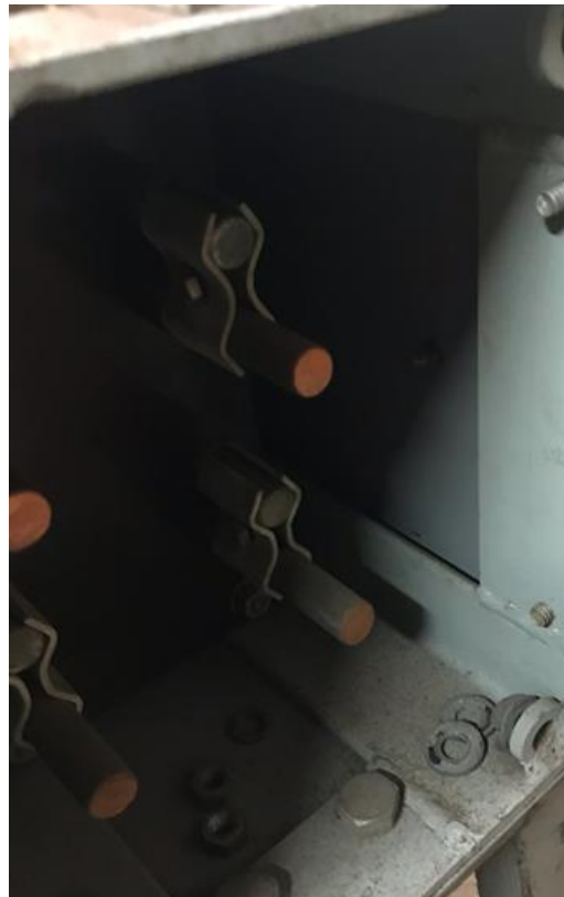
A close up view of the energised busbar and how close to the end plate they are.
