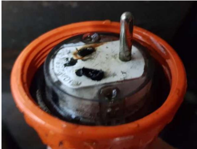
The IP56 rated plug with both the active and neutral pins missing, showing the heat affected areas
