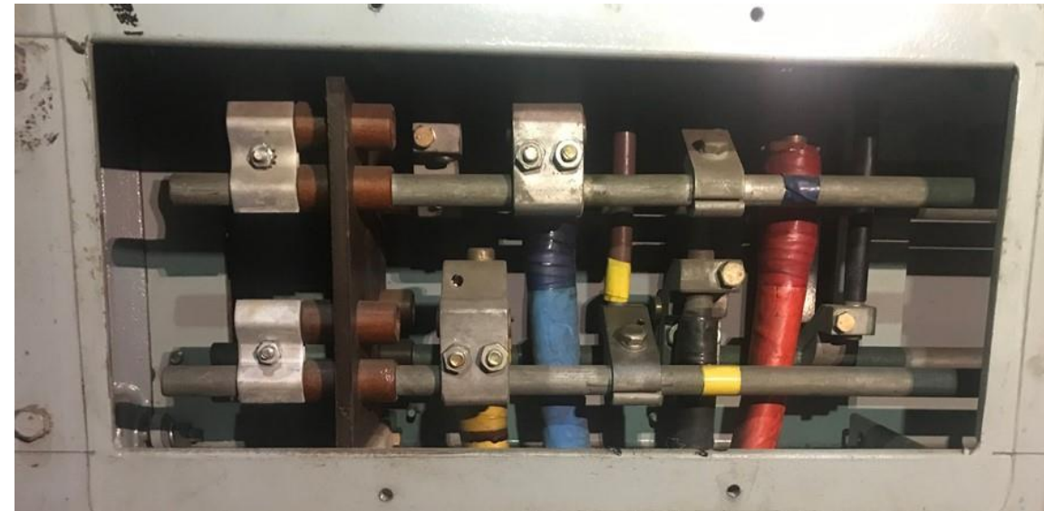
A side view of the CFS board busbar after isolation and covers were removed to secure the end plates
