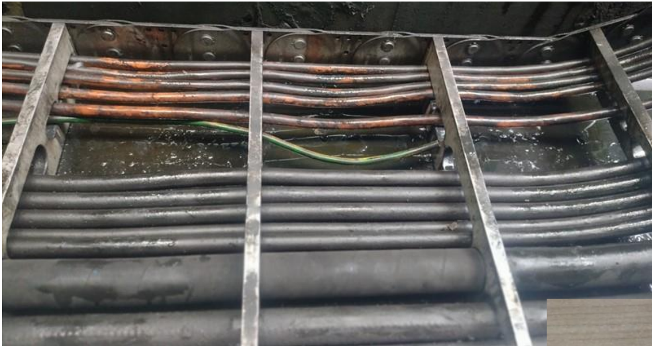
The metal cable chain, power cables and hydraulic hoses (bottom). Cables installed in the chain are normally exposed to oil.
