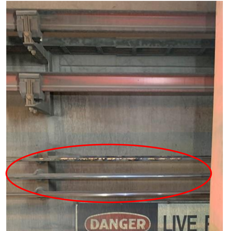
The damaged AC live rails
