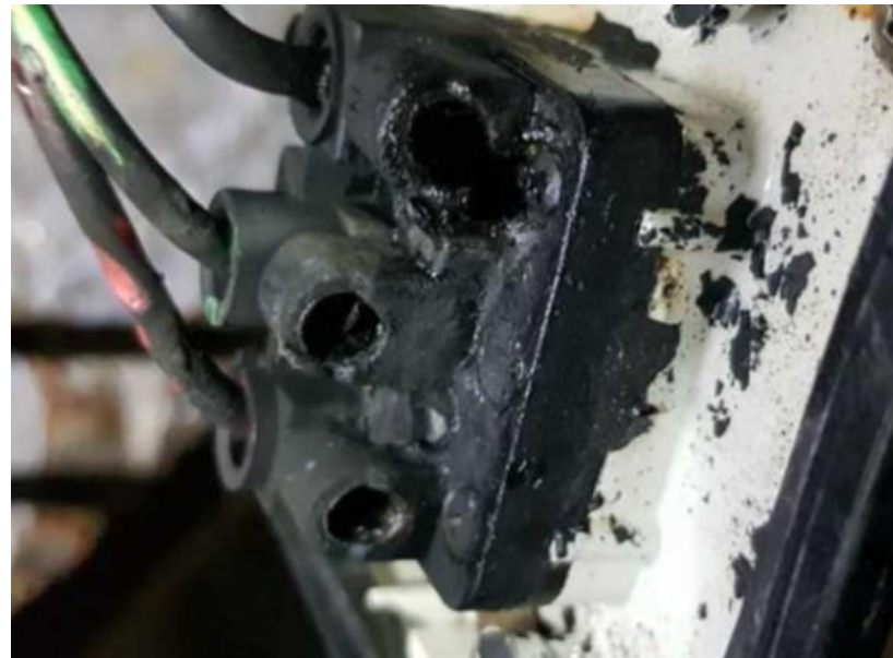
The inside of the socket outlet where the water has created a short circuit and hot joint between the active and neutral connections
