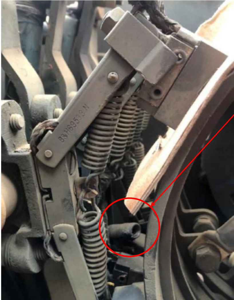
The arrangement of the 415V ac slip rings. The failed spring after it has caused the short circuit
