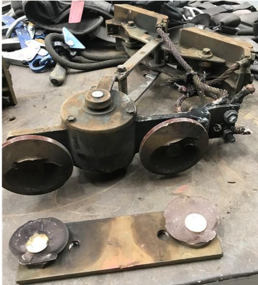
The middle phase collector shoe with both supporting insulators cracked and failed. Note all the melted pig-tails and burnt arms
