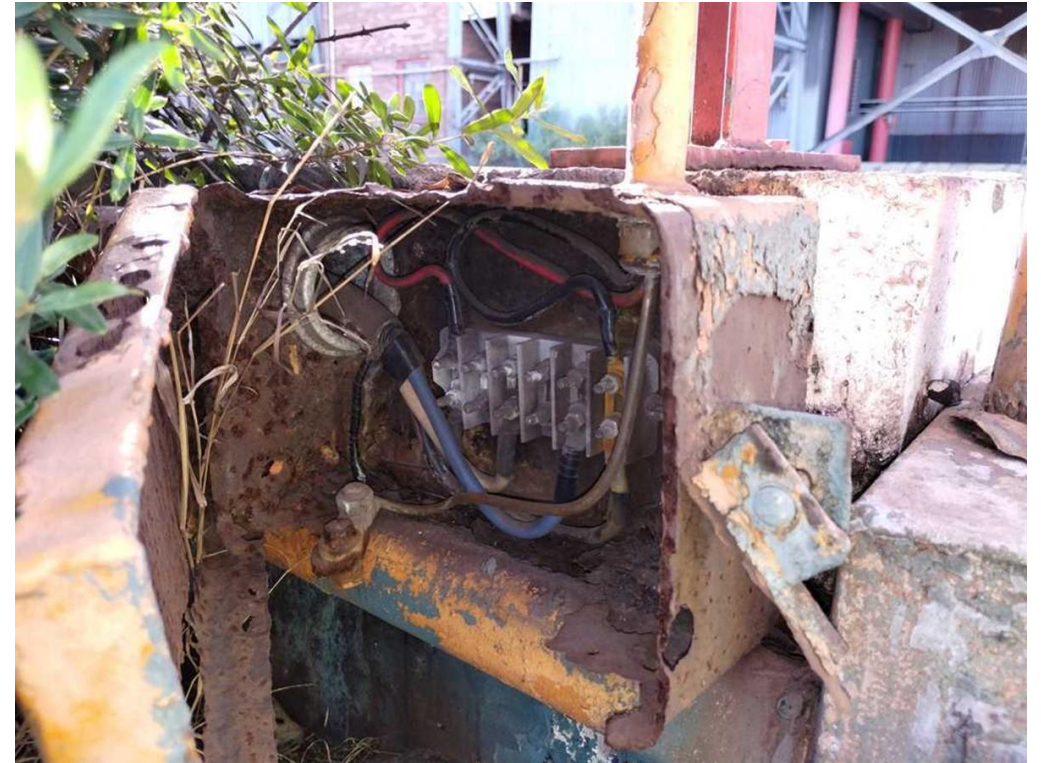
Nearby Steel Junction Boxes
