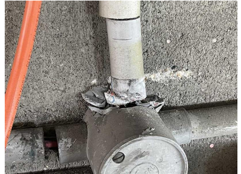
Damage to conduit and junction box below
