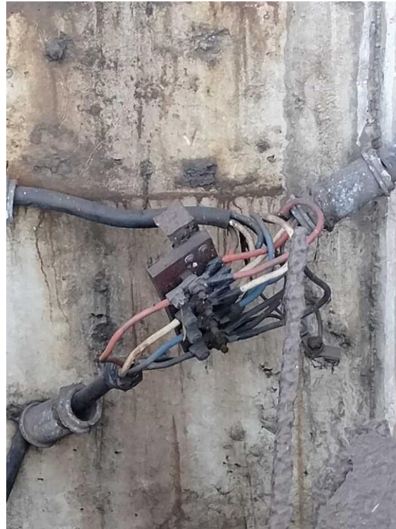
Exposed wiring inside pit
