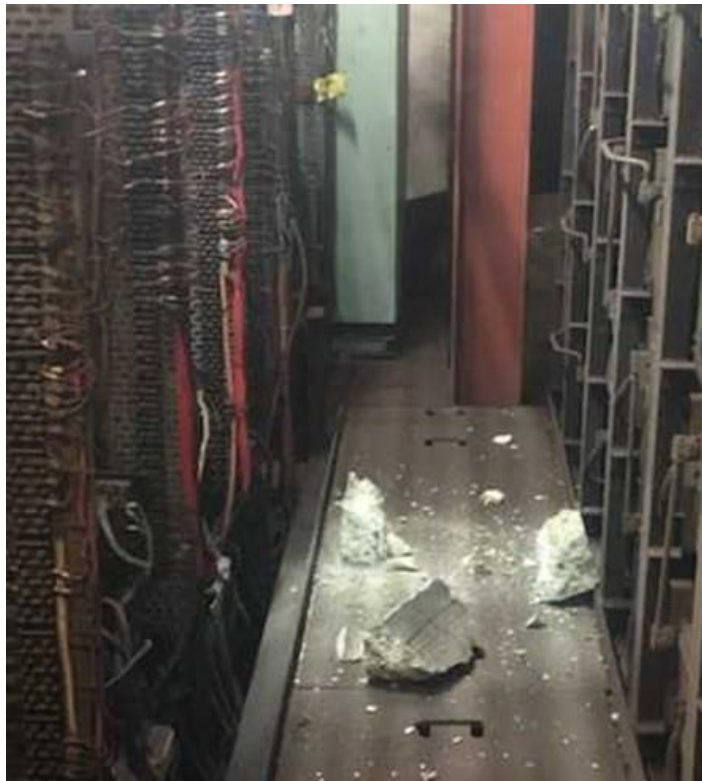
Concrete pieces behind electrical panels
