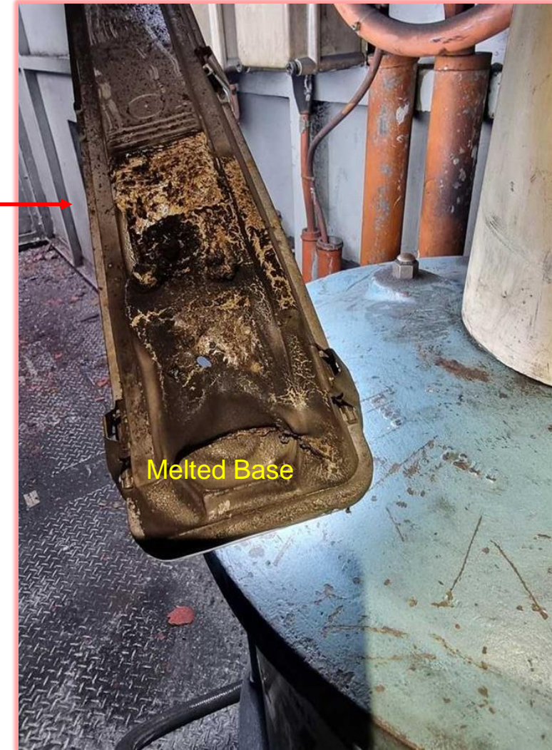
Damaged roof light
