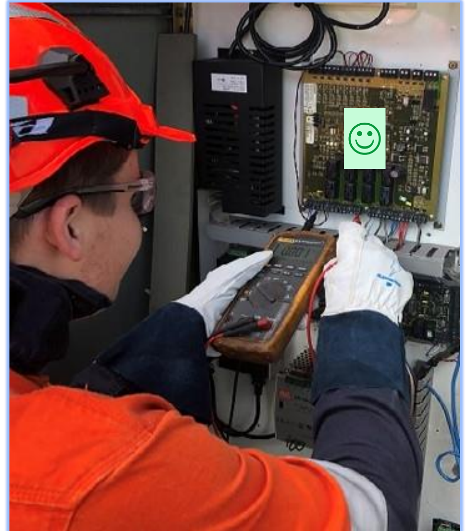
Example of Test Before You Touch being completed before working on an electrical panel.
