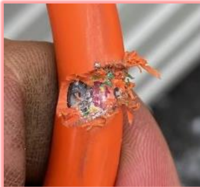
Cable damaged by hole saw
