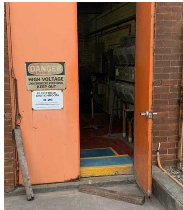
Door chocked open with timber
