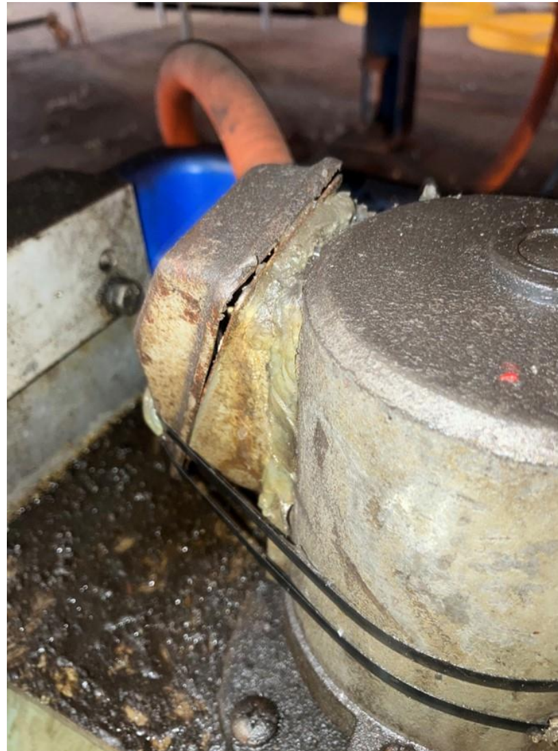
Motor terminal box IP rating insufficient for wet environment and cover not adequately secured
