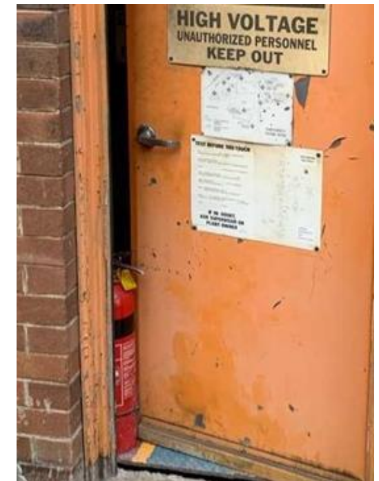
Door chocked with fire extinguisher
