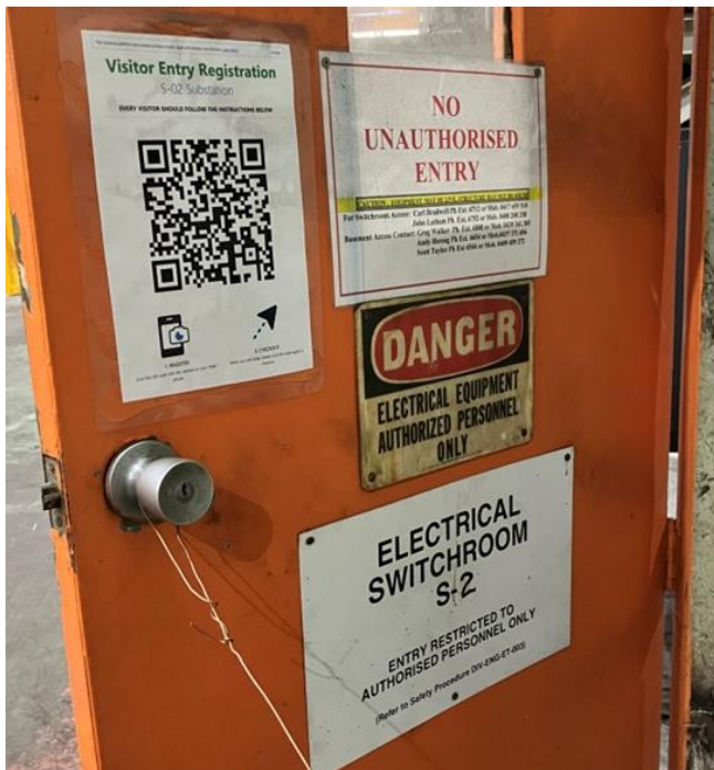
Door tied open with electrical cable
